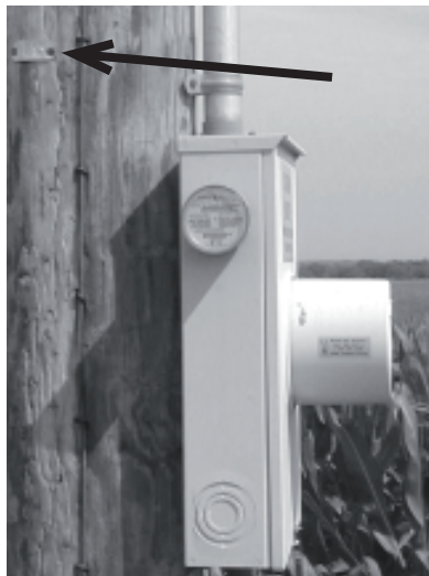
Well number on meter pole
